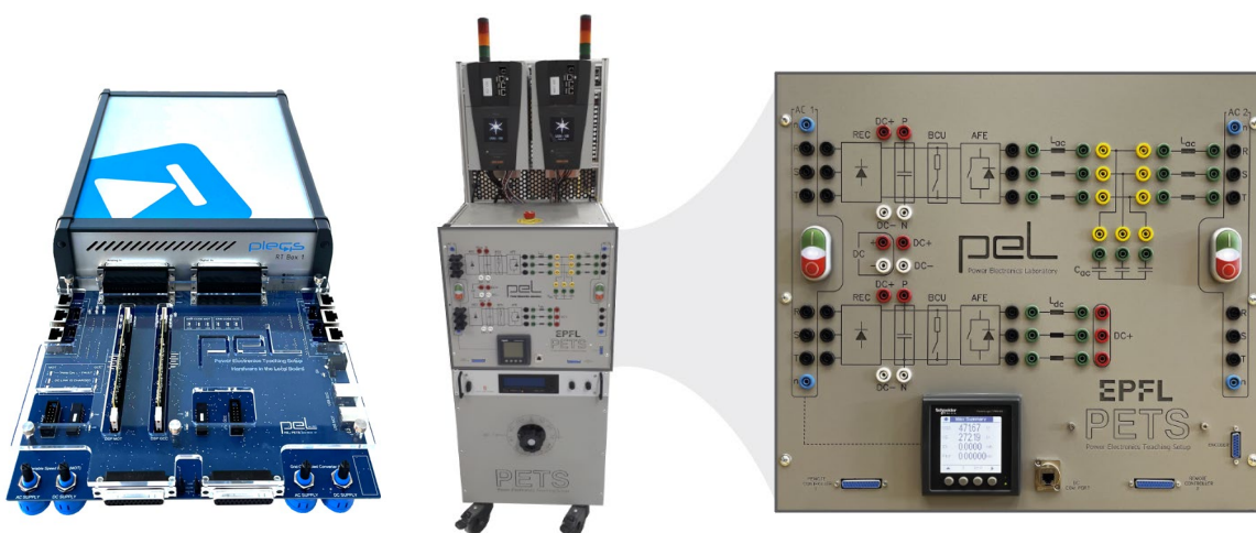
Fig. 1 PETS HIL (left) and actual PETS (right) that will be used for RT-HIL simulations and experimental investigations.
